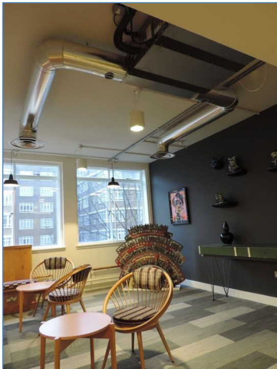
BELOW: All of the building services are on show including this Lossnay heat recovery ventilation unit.
